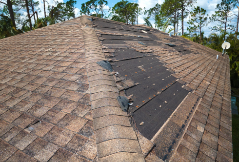
Missing shingles on a roof
