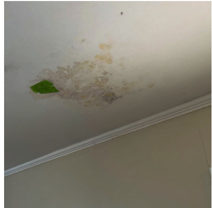
Ceiling stain indicating a roof leak
