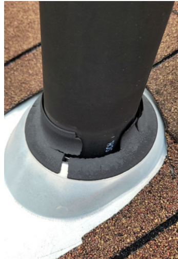
Cracked pipe boot
